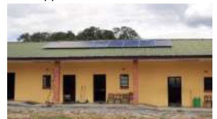
Solar panels on the Arise roof getting lots of sun
